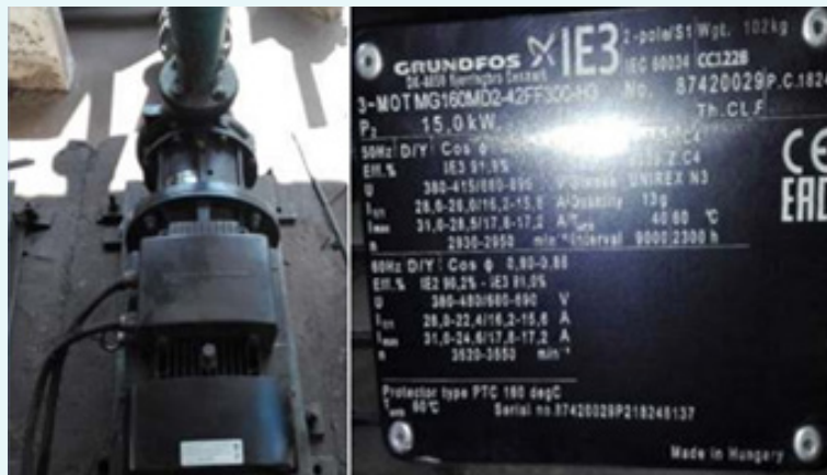
New EE Pump at Integra Automation
