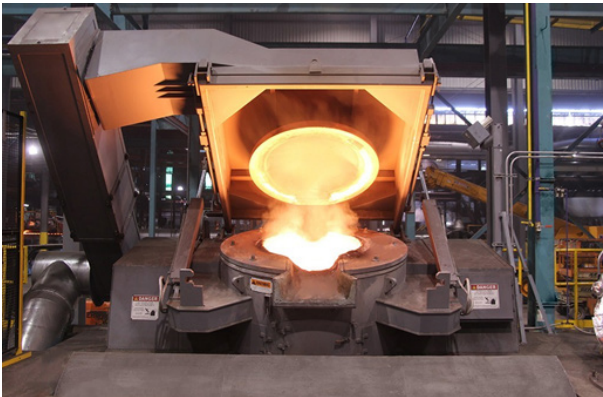
Figure 19: Lid Mechanism in an Induction Furnace
